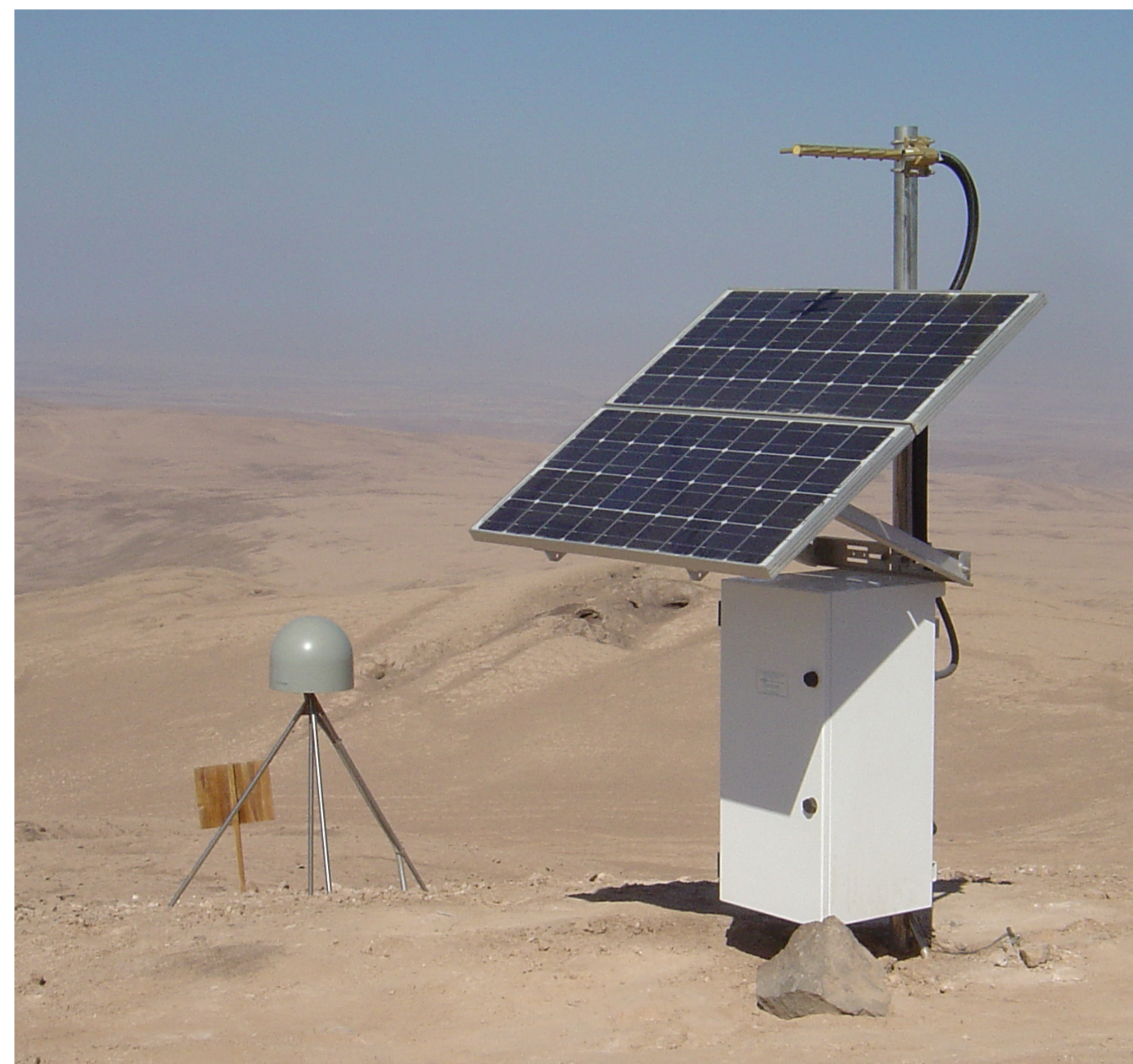
Figure 5. CAGA station ATJN in northern Chile. Equipment box, solar panels, and ethernet link radio antenna in the foreground, GPS tripod and antenna in the background.
