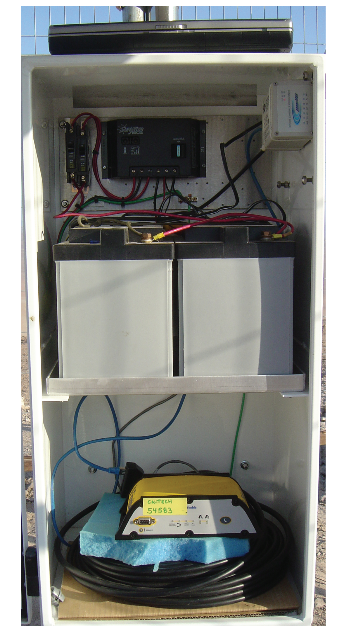
Figure 7. Interior of equipment box for station PCCL. Solar panel control unit and ethernet radio located above batteries, GPS receiver below.
