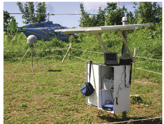
A typical GPS installation. The gray dome on the tripod in the background houses the GPS unit proper, and the open cabinet under the solar panel contains the electronics.
