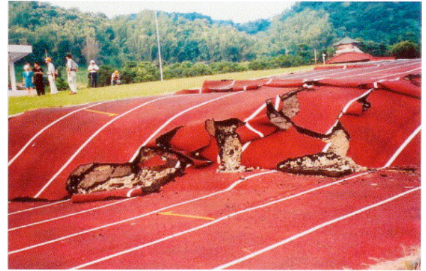
Fig. 7. View of the flexural scarp produced by the 1999 Chichi earthquake at Kuangfu Middle School sport ground. Overriding hanging wall on the footwall, and complex deformation on the hanging wall are clearly seen (Kuangfu Middle School sport ground, photo by Ota, September, 1999).
