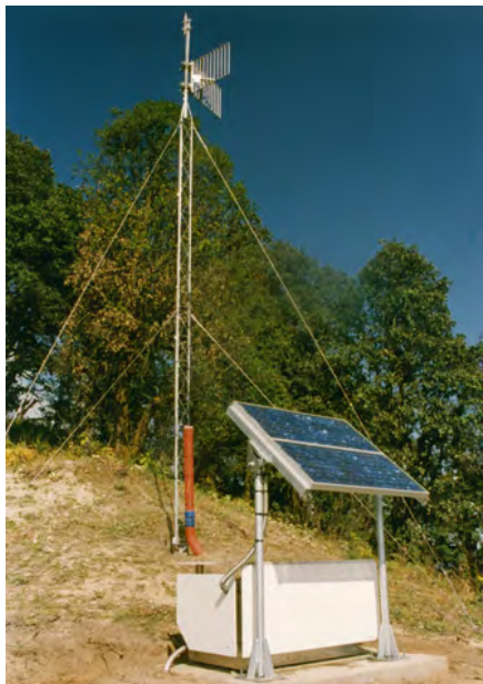
Seismic station antenna and solar panel
