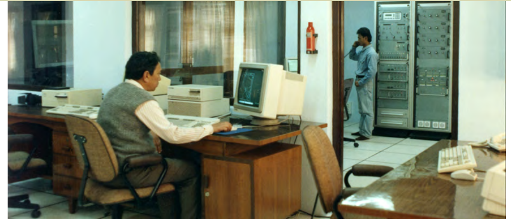
View of recording and processing center at NSC
